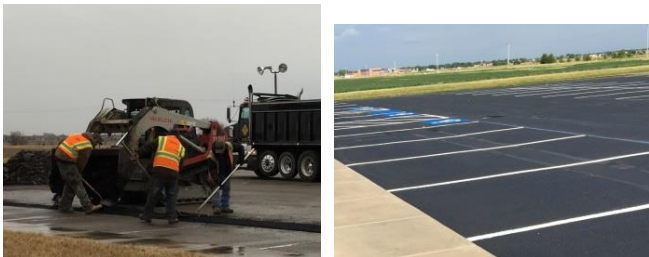
(Left) The HUGE crack has disappeared.
