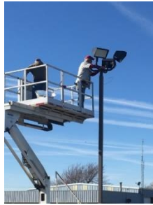
New LED lights installed
